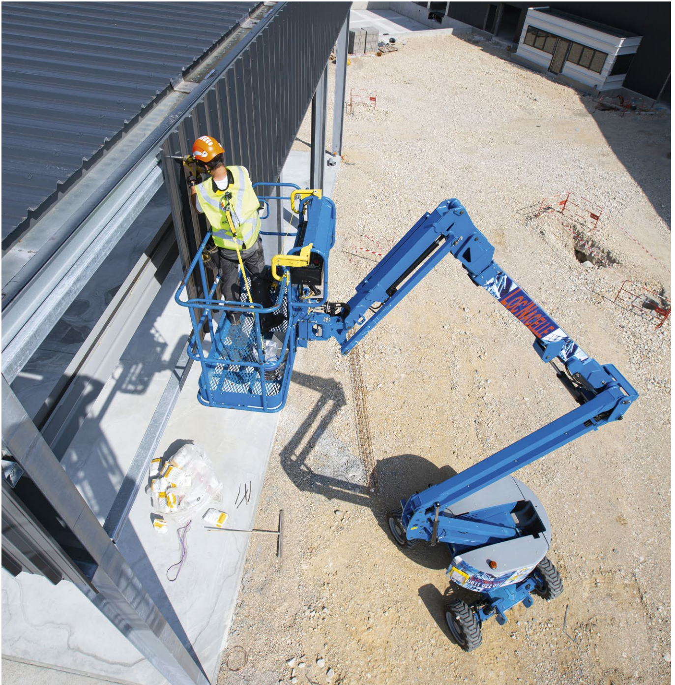
Working from an aerial work platform; Bourg-en-Bresse, France © 2020 Petzl Distribution - Lafouche - LOCNACELLE
